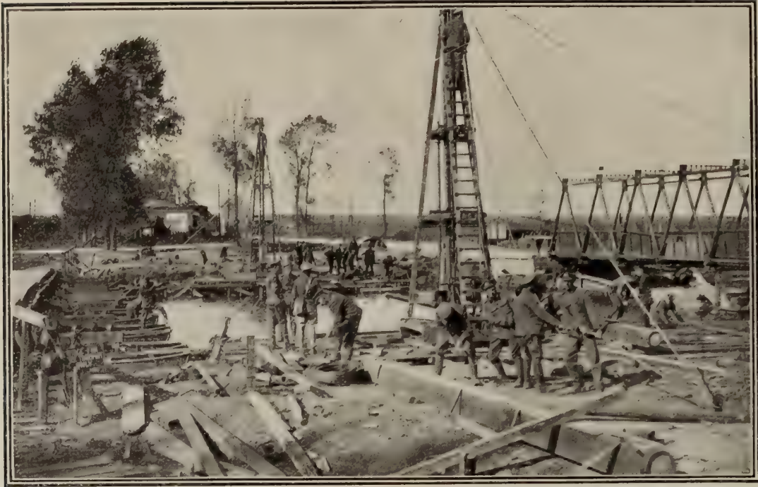
Canadian Engineers building an extra bridge across the Canal du Nord; the bridge on right was built by them in eight hours under heavy shell fire. Note pontoon bridge on left.
